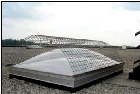
Example of a skylight with safety cover
