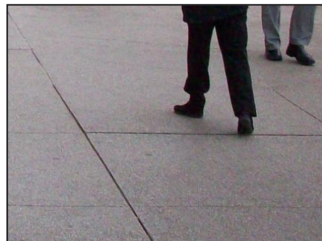
Sidewalk slabs float, creating trip hazards.
