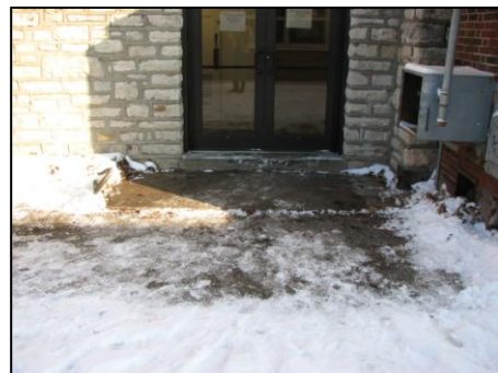
The condition of this doorway is unacceptable. Clear snow and ice.
