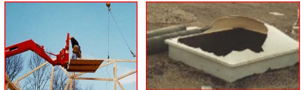
Skylights are holes. Cover them!
