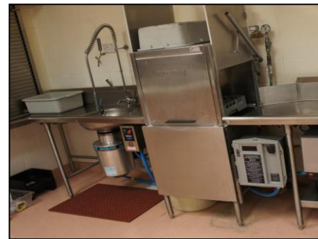
Sink areas are almost always wet, creating slip hazards.
