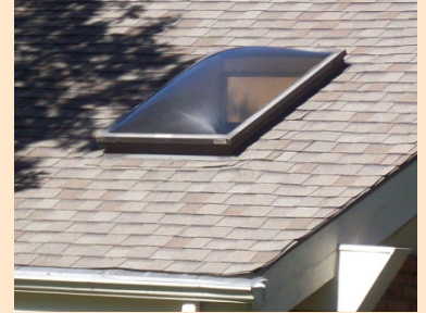
Skylights must be protected when employees are on the roof.
