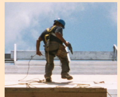
Unsafe: This employee is not tied off.
