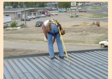
Correct: This employee is using a personal fall arrest system for protection from a leading edge fall.
