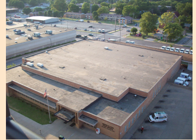
This flat roof can expose roofers and HVAC employees to a leading edge fall hazard.
