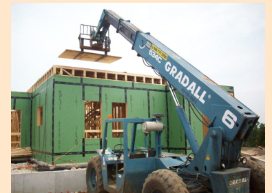
The second floor of this structure exposes employees to a leading edge fall.
