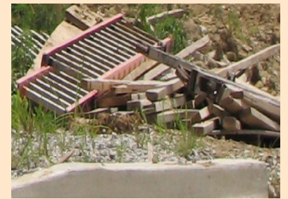
Unsafe: This ladder is thrown into the debris pile.
