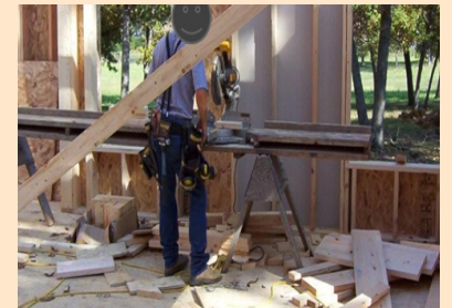
Unsafe: This work area is littered with scrap materials.
