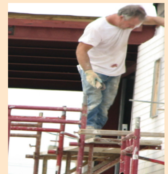
All scaffolds need guardrails.
