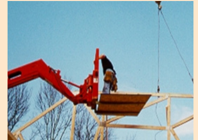
Lifting employees on the forks or in buckets can lead to a fatal fall.
