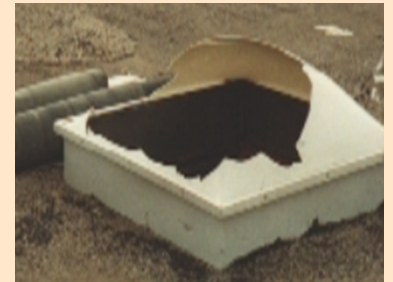
Cover all skylight holes.
